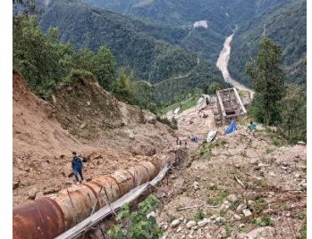
Penstock Pipe enclosed casing
